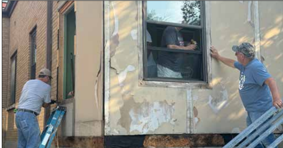
New windows were put in the church offices. New siding has begun.
